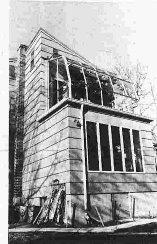
One side of an older duplex was extended in the rear to provide extra living room downstairs, and a luxury bath and green house upstairs.
